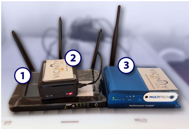
Figure 13: Routers/gateways placed on top of the refrigerator
