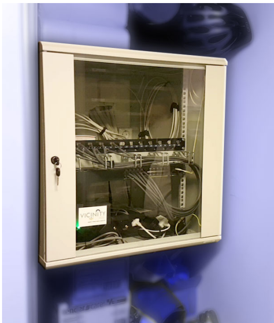
Figure 15: Locked steel closet for equipment
