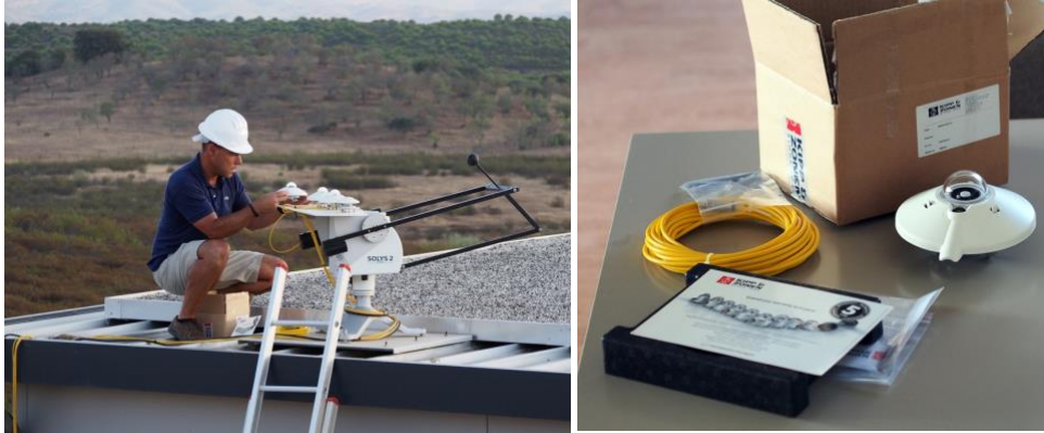
Figure 16 - UV radiation sensor installation at SolarLab
